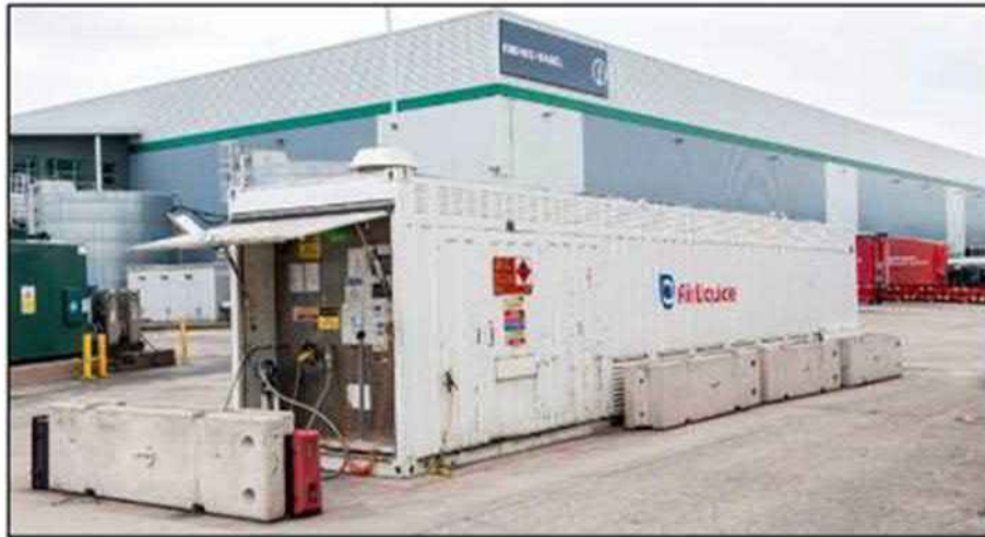
Figure 2-17: Typical containerised LNG facility
