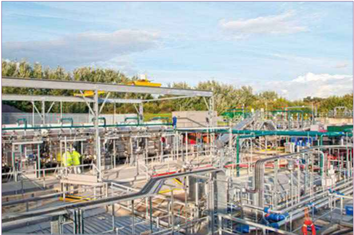
Figure 2-6: Mogden WWTP (West London) inlet works
