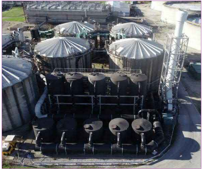
Figure 2-12: Hull STC Odour Control Plant
