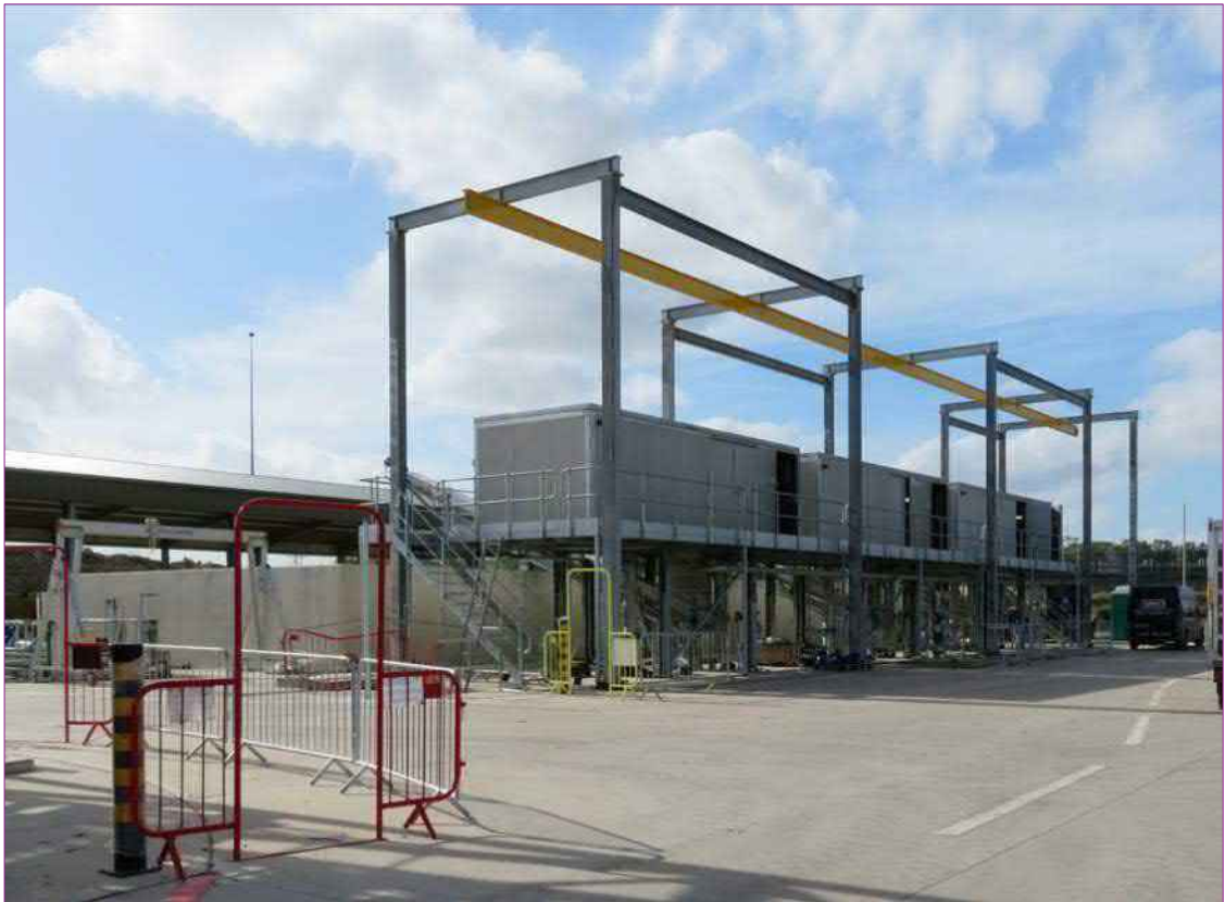
Figure 2-15: Sludge Dewatering at Knostrop sludge treatment centre
