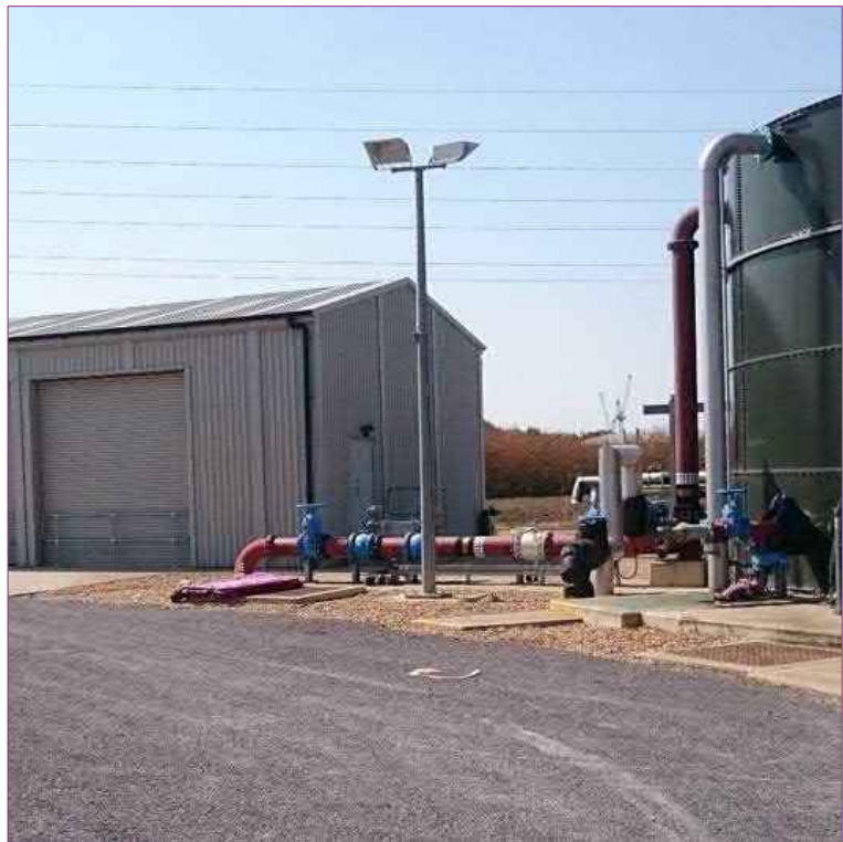
Figure 2-20: Example lighting unit
