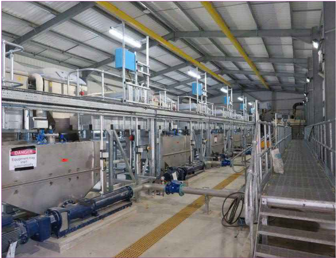
Figure 2-11: Thickening Building Knostrop sludge treatment centre
