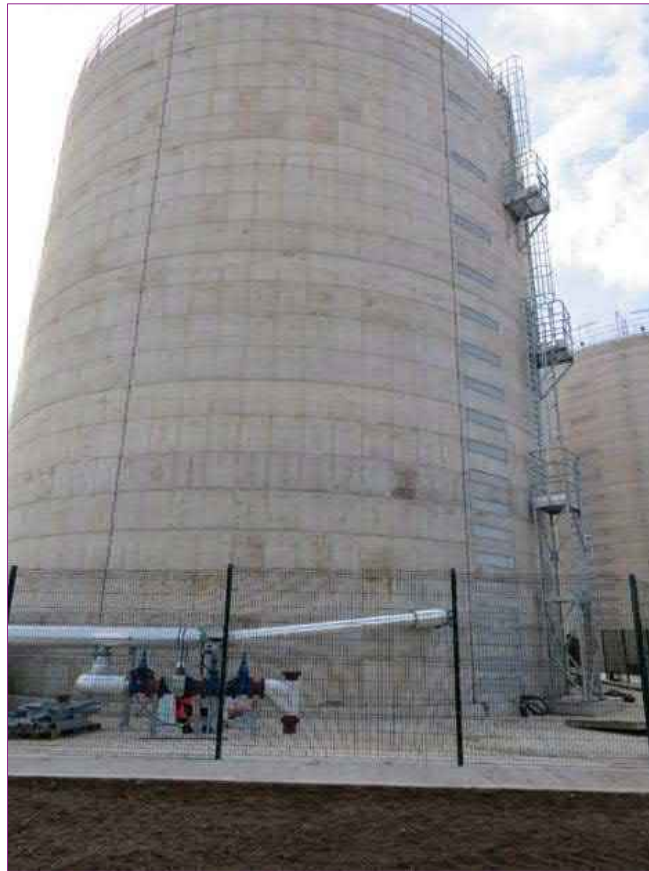
Figure 2-14: Digestion Tank at Knostrop sludge treatment centre
