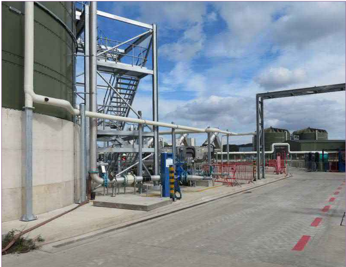
Figure 2-10: Sludge Imports Knostrop sludge treatment centre
